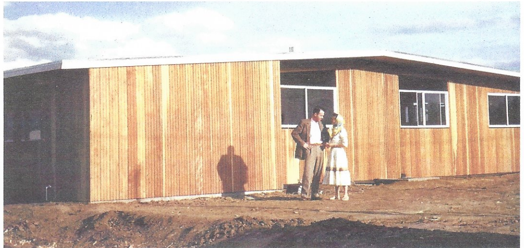
STEP BACK IN TIME. A month before their memorable July 4, 1955 move-in date, original owners Val and Elaine Senter (above) posed alongside their new Wolff home under construction. The couple still lives there today. Admired by artists, architects, and other professionals, these homes now sell for $300,000
